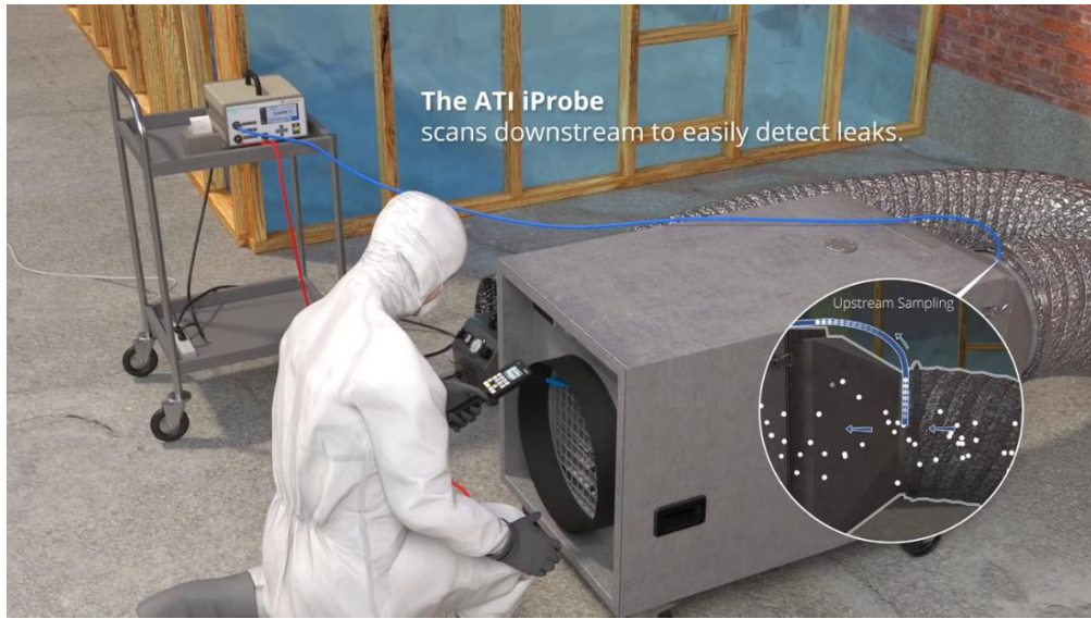
4 Field technician testing for leakage through the HEPA filter as part of the performance leak testing.
